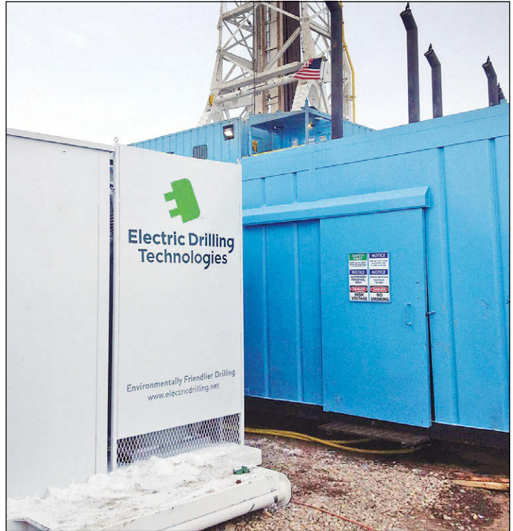
EDT feeds electricity into the Continental rig.
